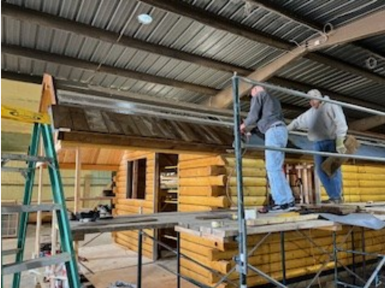
More progress pictures! Working on the cedar shake roof for the cabin that will be going to Glacier Camp
